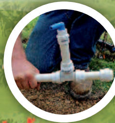
Irrigatie Flow Control
