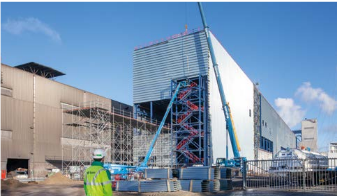
Aperam foundations for two new production units, Genk (Belgium) - BAM Contractors bv
